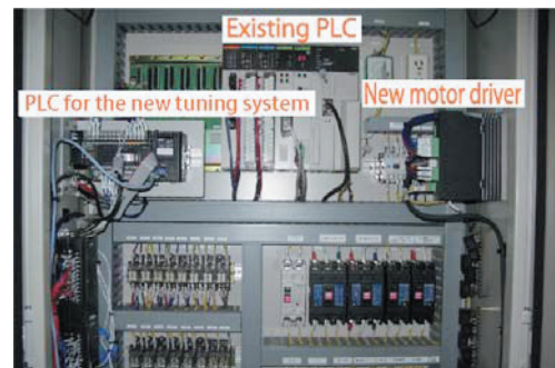
Fig. 2. Control unit of the new tuning system built in the existing RF control system for RILAC cavity 5.
