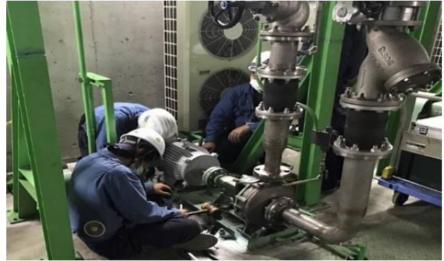
Fig. 1. RIBF water-cooling pump maintenance (Periodic maintenance).
