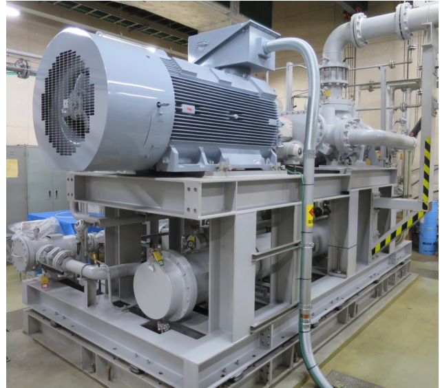
Fig. 2. Compressor unit with the new motor.
